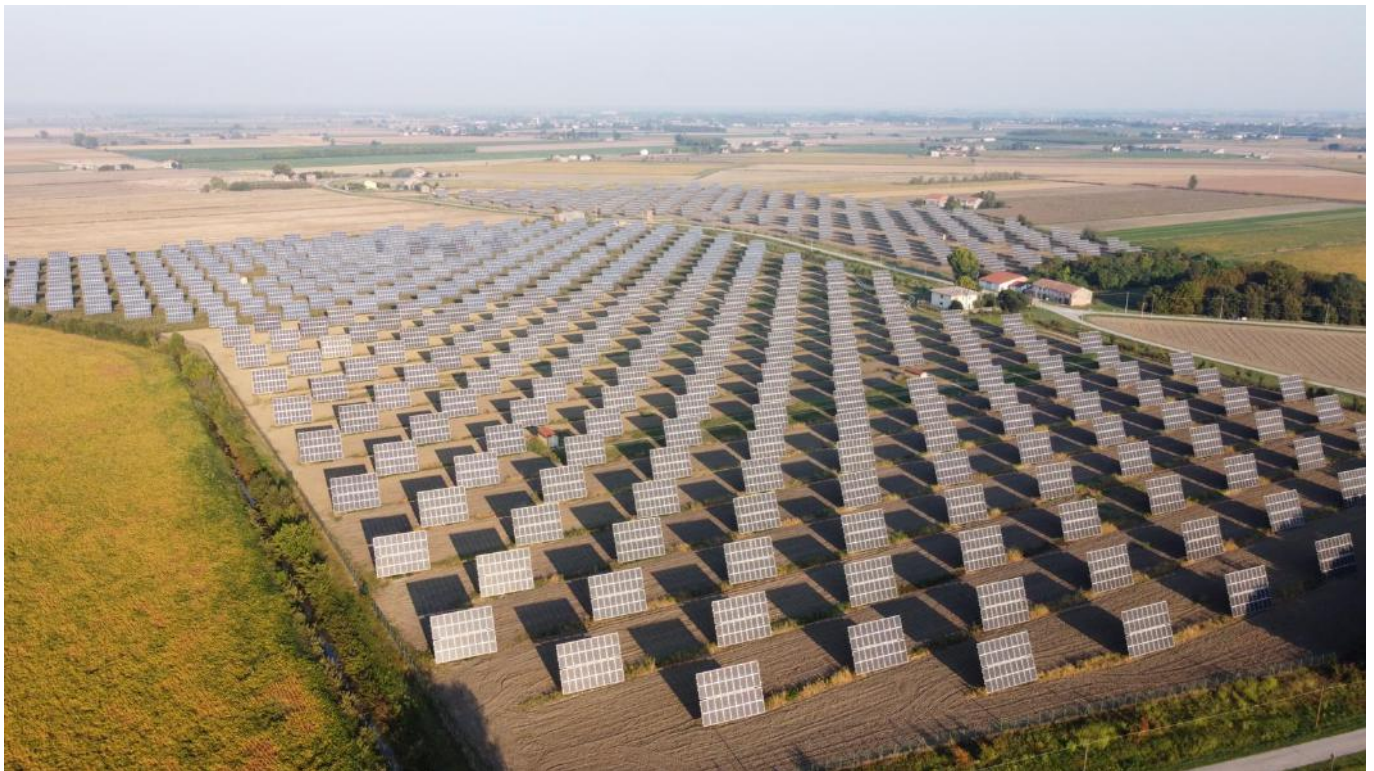
The solar power installation in Castelguglielmo has been fitted with more efficient bifacial modules.
