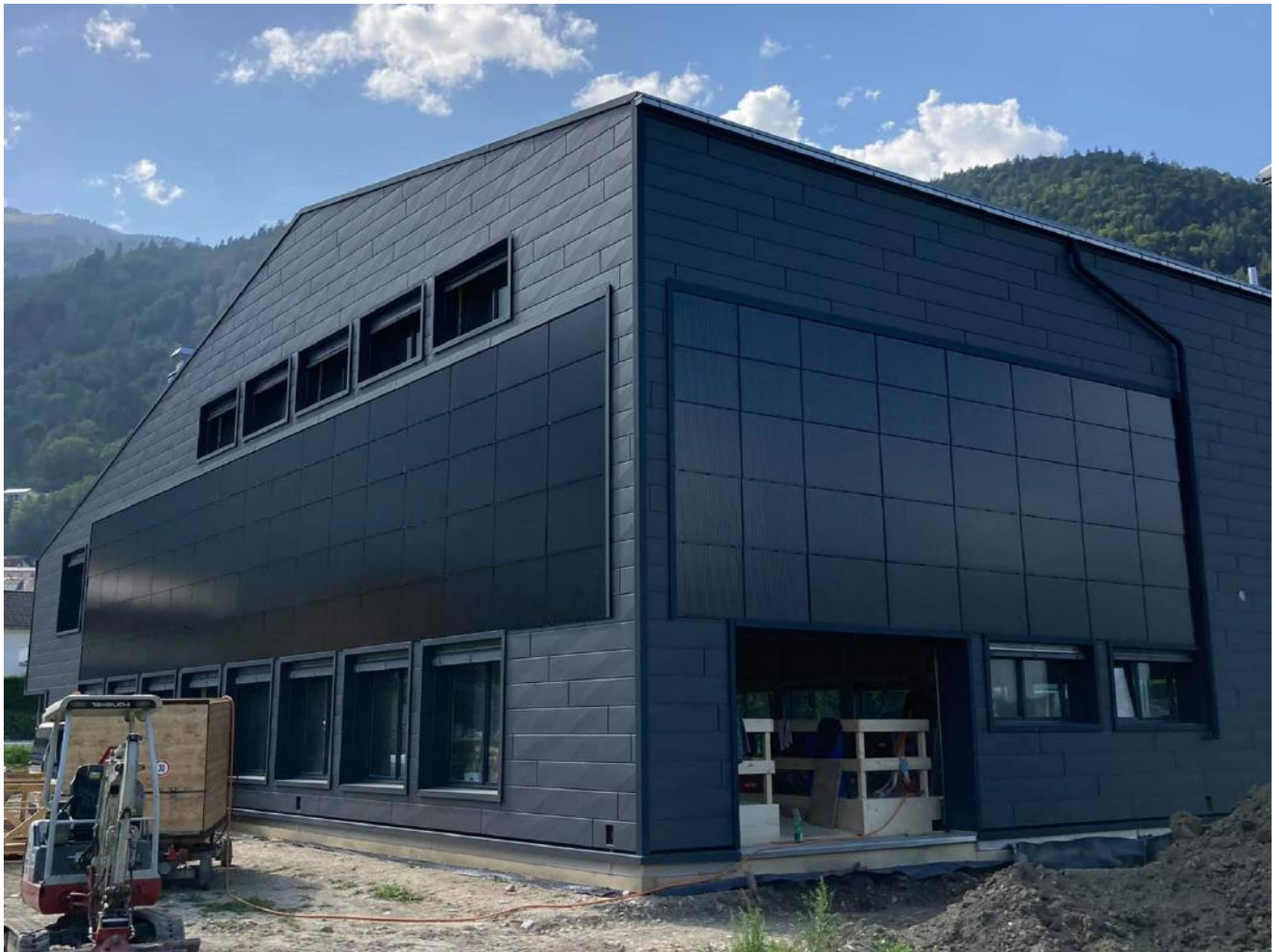
The roof and frontages of the new Rüfeli wrestling and sports hall in Untervaz have been fitted with a solar power installation from Repower.
