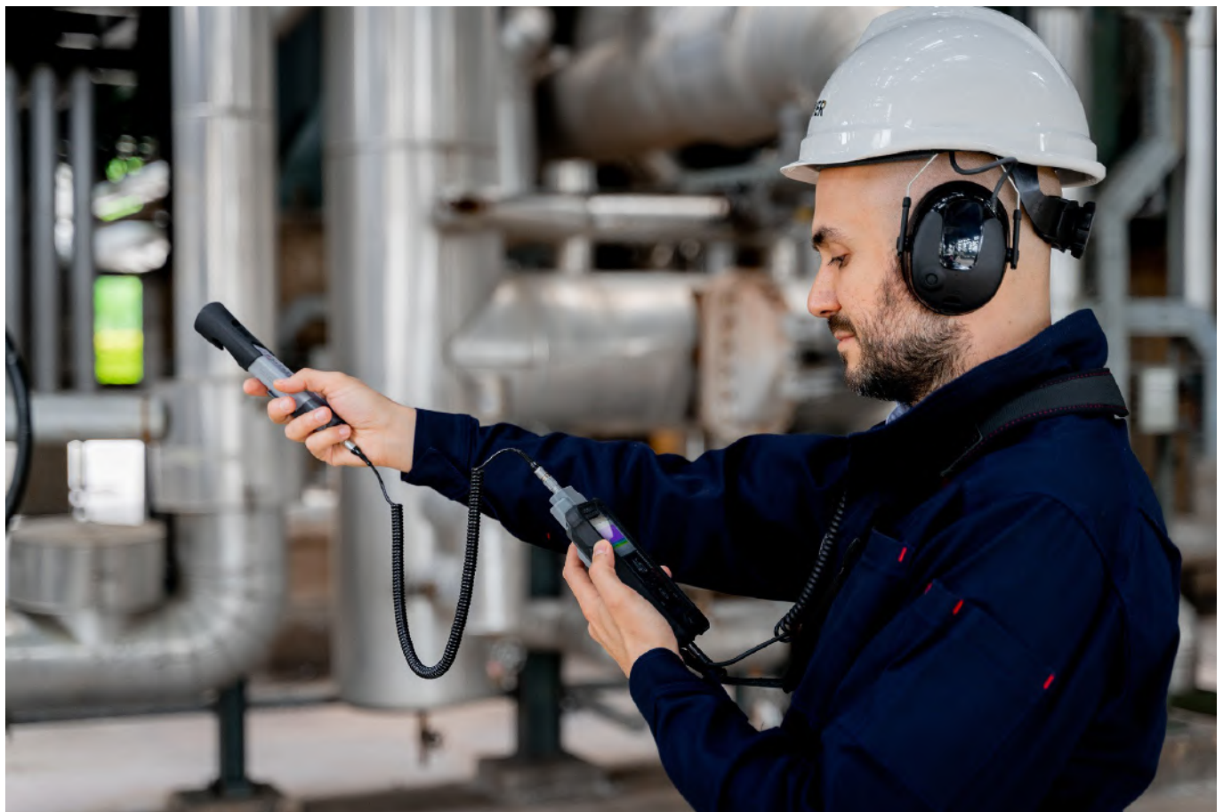
A Repower employee listens to a customer's compressed air system for possible leaks.
